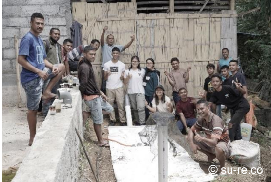
Biogas installation in Bajawa
